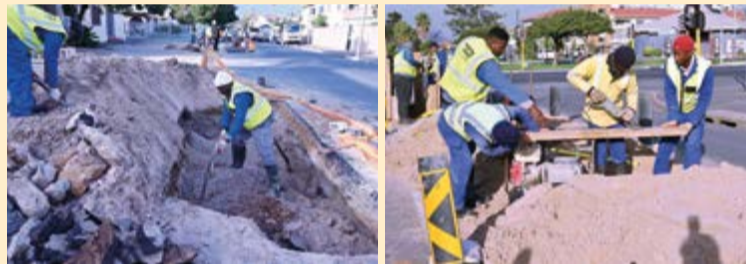
Dig, replace, repeat: The City's teams are diligently following their schedule of proactive water and sewer pipe replacements across town to minimise the risk of pipe bursts and improve overall water and sanitation services.
